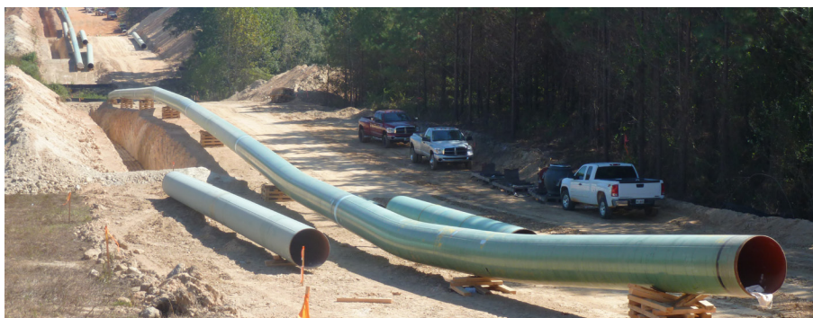
Stringing the pipe in Coosa County, AL, as part of Phase II construction of our 85 North Expansion project.
