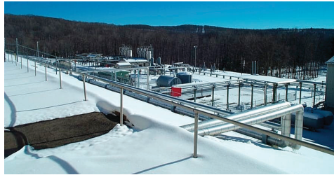
Snow covers Station 535 in Pennsylvania
